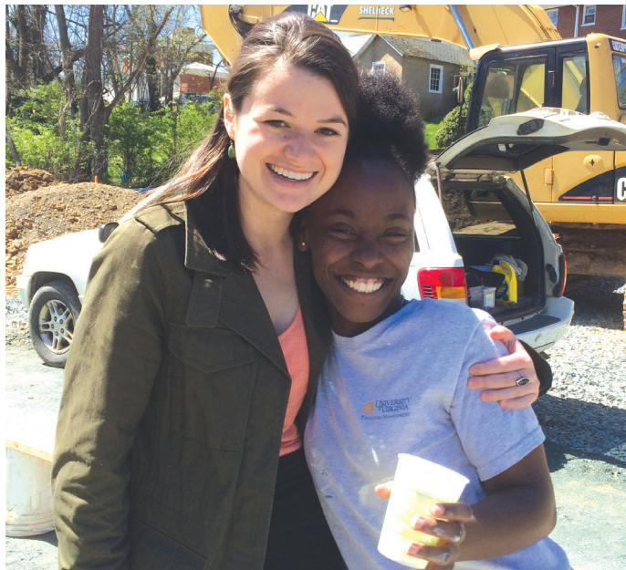
Habitat Youth United Coordinator Lydia Prokosch joined new Partner Family Angel Turner for an exciting first day on the construction site.
